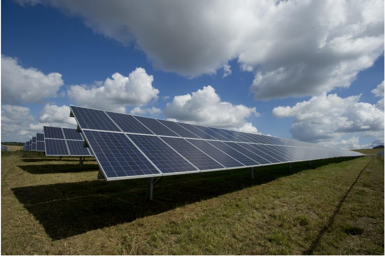
Solar Panels placed in five acres of land owned by the institution
